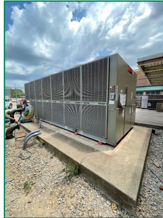
New Chiller for KCAL
