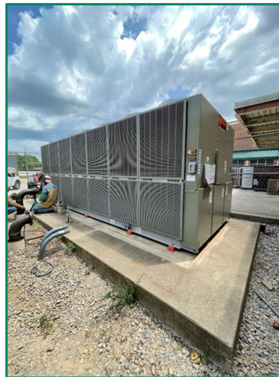
New Chiller for KCAL
